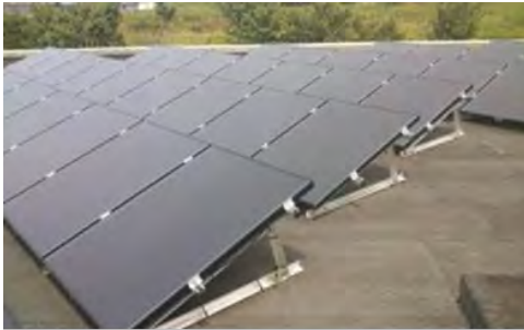
Photo Voltaic panels on the roof of the school
